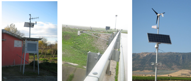
Figure 5 Periphery sensor system
